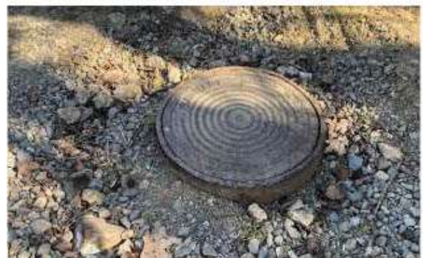
Problematic Manhole in Regan Road
